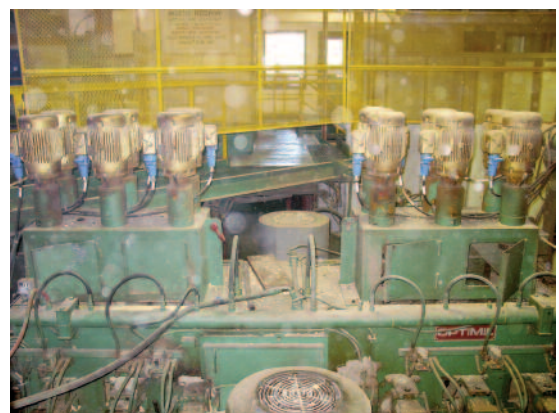
Closeup shows typical motors with Meltric Decontactors in place. Dead-front construction keeps workers safe, while plug-and-play simplicity speed motor removal and reinstallation.
