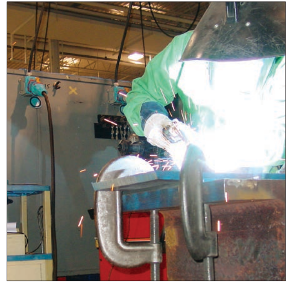
Three MELTRIC Switch-Rated welder receptacles provide power for Gas Metal Arc Welding (GMAW) in an EWI work cell.
